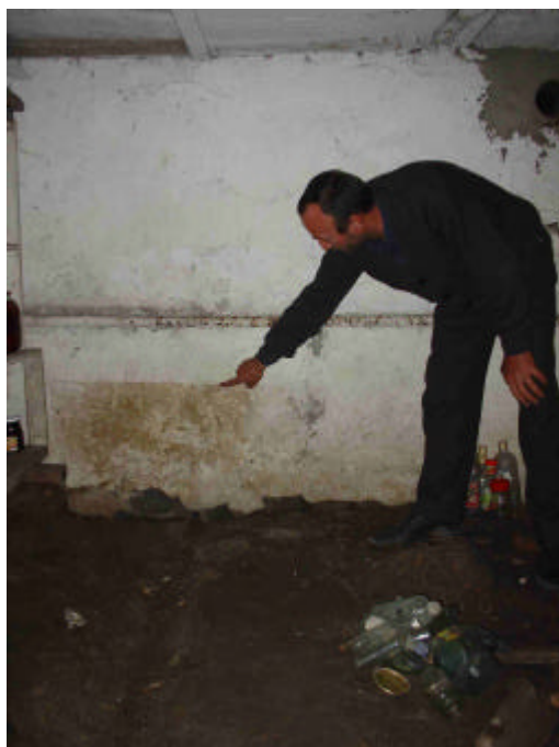
Edna Abuladze shows the Mission evidence of the flooding in his basement.
