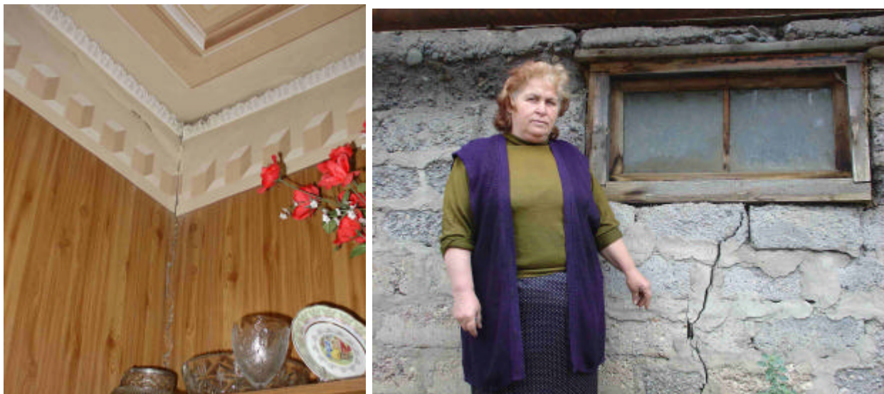
Mrs Lomidze claims intense heavy traffic has resulted in damage to her house. Left: One of Mrs Lomidze recently cracked walls inside her house. Right: Mrs Lomidze indicating damage outside her house by vibration pollution of BTC traffic.
